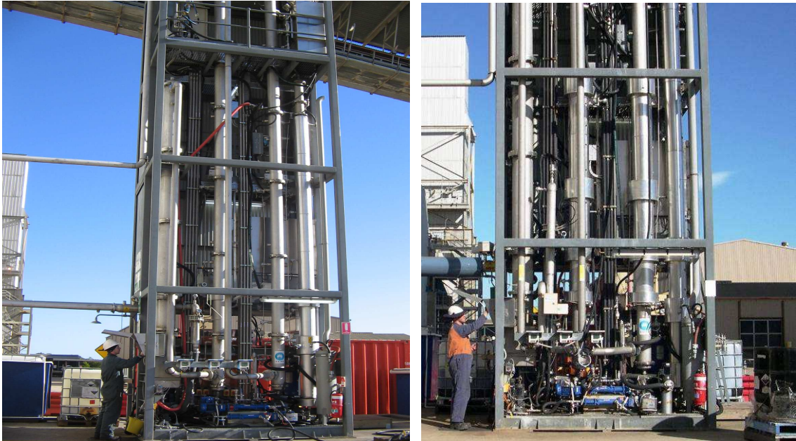
Figure 33: CSIRO's PCC pilot plant at Loy Yang Power (2008 left and 2011 right).
