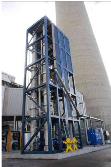
Munmorah – since '09 Black coal-fired power station
