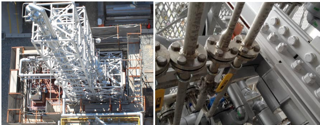
Figure 7 Design to completion – Birds eye view PICA plant (left), Well supported pipe-lines with break-line flanges to facilitate module separation (right).
