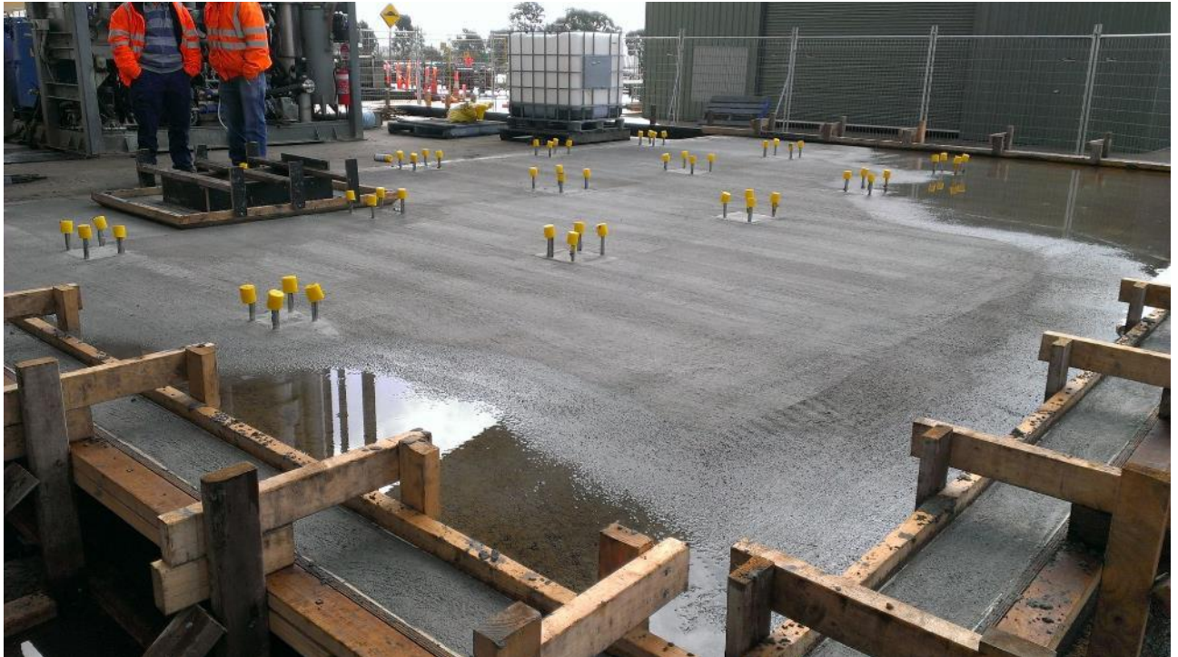
Figure 8 New slab adjoining old slab. Hold down bolts for pilot plant built in position.
