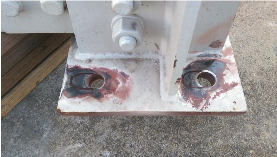
Figure 13 Structural engineer approves elongated bolt holes and later steel plate reinforcing
