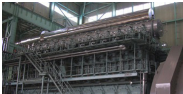
Figure 8 - A mid-size low speed engine with generator by MAN (55 MW, 120 rpm)
