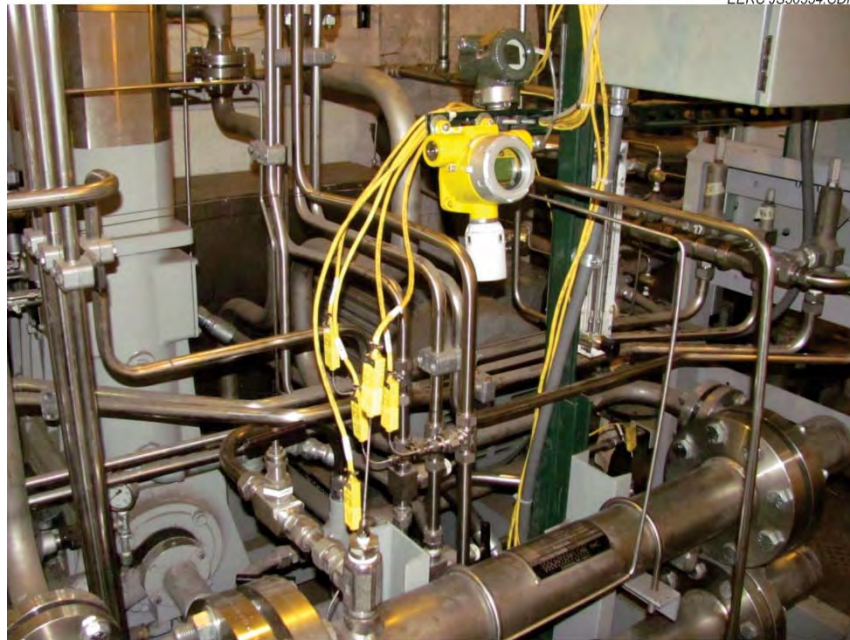
Figure 28. Instrumentation added to the syngas compressor.
