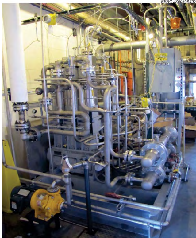
Figure 25. Hot-syngas compressor skid.
