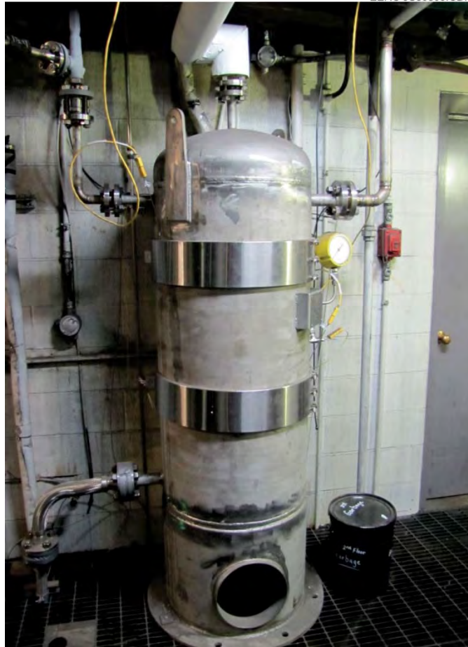
Figure 27. Compressor surge tank.
