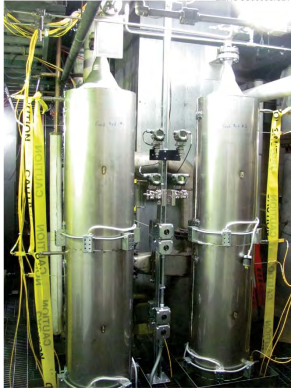
Figure 32. Sulfur capture fixed beds as installed on the second floor of the TRDU tower.
