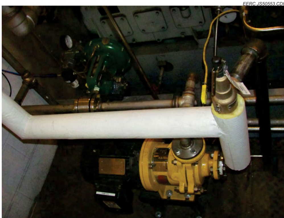
Figure 29. Modified coolant pump and control valve.
